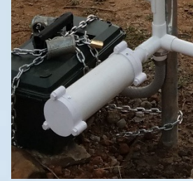
Data Logger Housing
